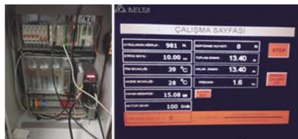
Fig. 2. Appearance of cabinet for electronic equipment and Control Panel working page.
